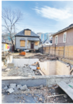
The Upton residence moved off its foundation. Image courtesy of Christie Page.
