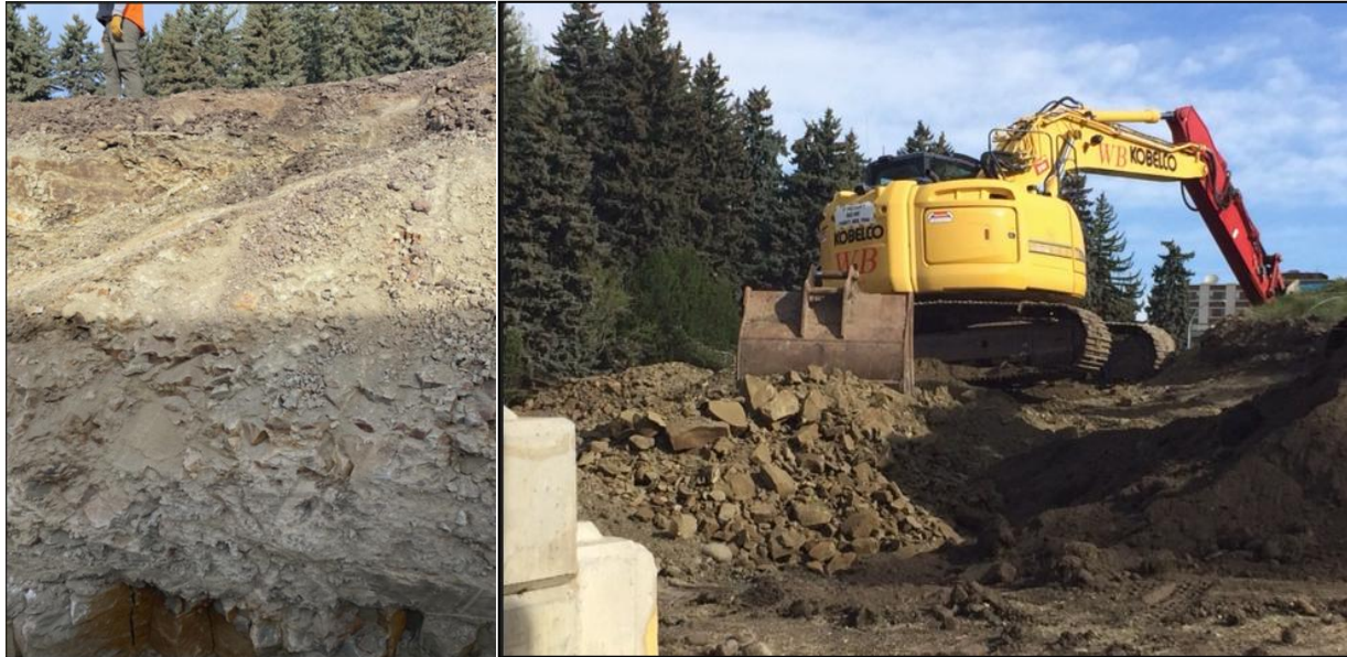
Figure 19. Excavation pit photo at base of 10th St. N.W. hill for the upper plateau storm water diversion tunnel. The very bottom of photo on left shows pit walls of yellow coloured sandstone below grey coloured claystone. Photo on right shows yellow sandstone rubble lifted out of pit. Thanks to Theo, site supervisor, for photos.
