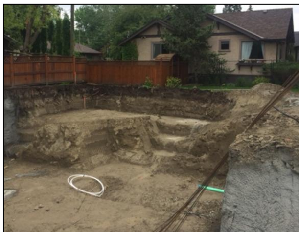
Figure B3. Sandy glacial lake sediment in a 2022 house excavation at 6A St. N.W. and Alexander Crescent. No evidence of Mazama Ash in this photo.
